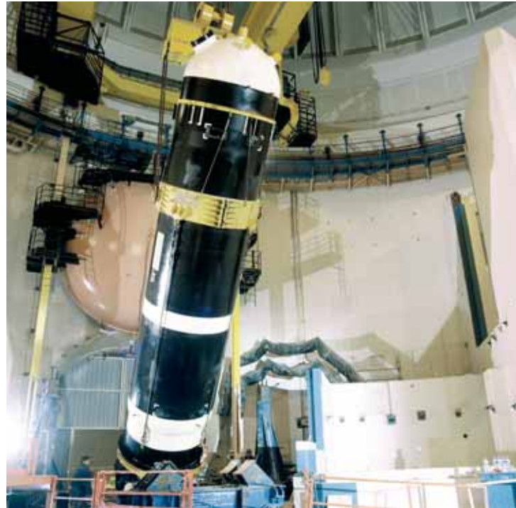
Pressurizer being rigged into place at the French nuclear power plant unit Golfech 2. The pressurizer for the EPR will be 14.4 meters high and will weigh around 150 tons when empty.
