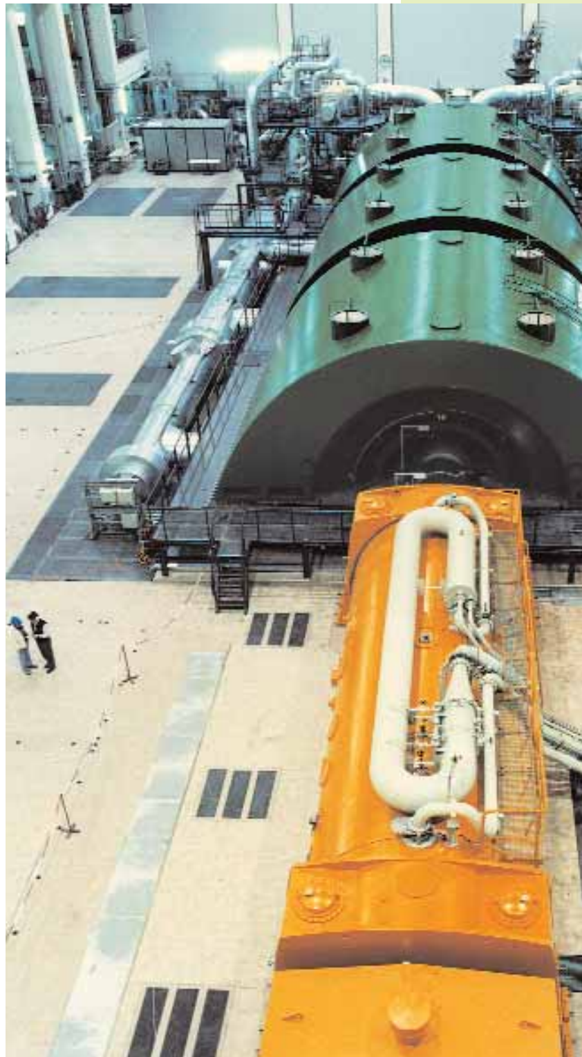
Turbine generator set at Isar 2: the exciter and the generator are in the foreground
